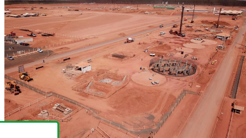
White liquor plant
